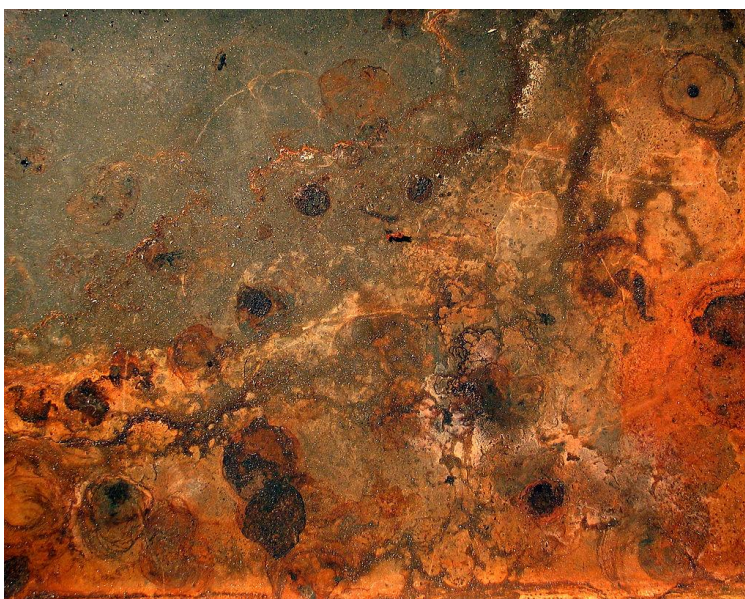
Fig. 15. Rust-The most familiar example of corrosion
