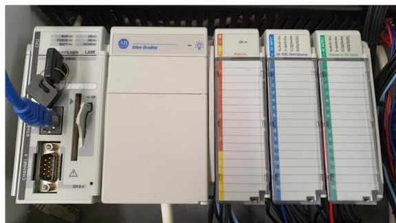
Fig. 5: Allen-Bradley 1769-L32E PLC
